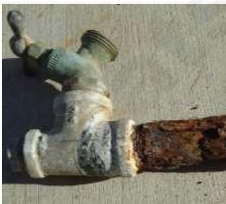
Copper alloy fitting connected to a galvanized iron fitting
